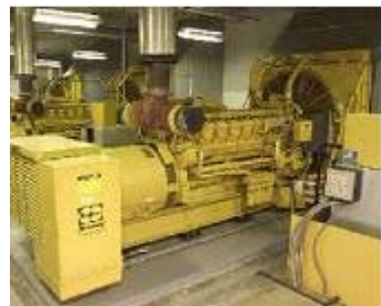
AITC Back-Up Generators
